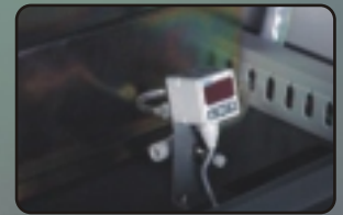
Negative Pressure Control
